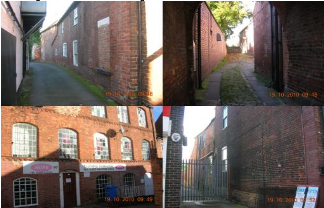
Figure 3.20: Top left: Rear of 14 Park Street. Top right: White Hart Yard. Bottom left: Building within Forrests Yard. Bottom right: North elevation of 79 Bridge Street.
