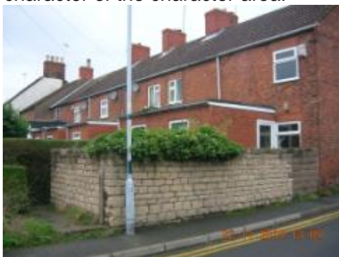
Figure 3.127: View of stone wall to rear of No.22 Canal Road (part of an earlier building).
