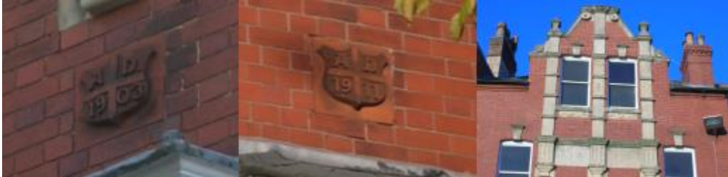
Figure 3.36: Left and centre: Terracotta inserts with the dates “AD 1903” and “AD 1911”. Right: Stone detailing on second and third floor, facing Bridge Street.
