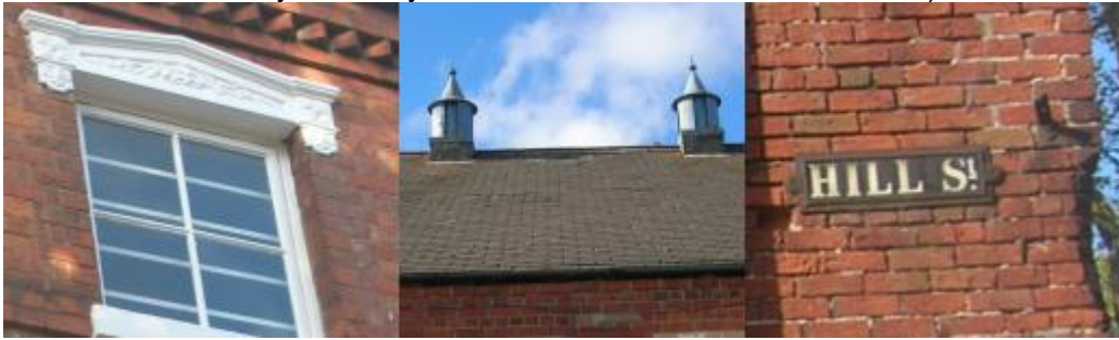
Figure 3.44: Decorated window header at 78-80 Bridge Street; Centre: Cowl ventilators at Worksop Bowling Club, Newgate Street; Right: Minton tile street name plate at Hill Street.
