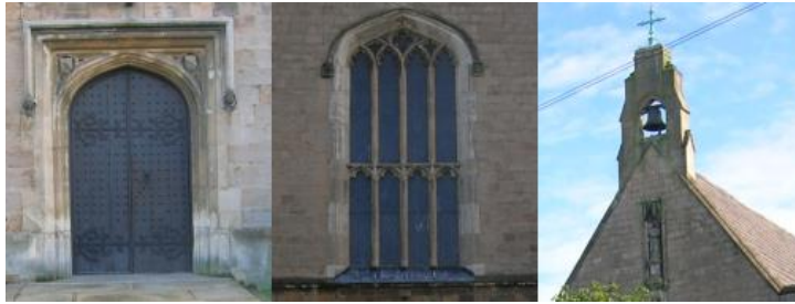
Figure 3.38: West elevation features including door (left), windows (centre) and bell cote (right).
